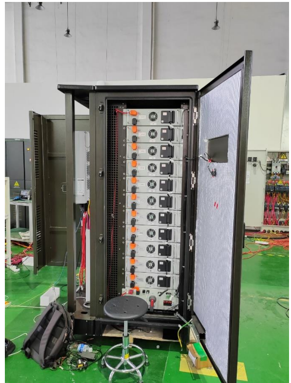
Front view of Battery system
