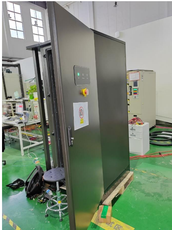
Side view of Battery system
